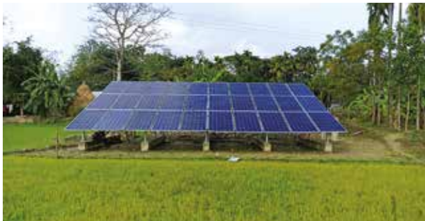
Figure 1: Solar Irrigation Pump at Kishoreganj PBS
